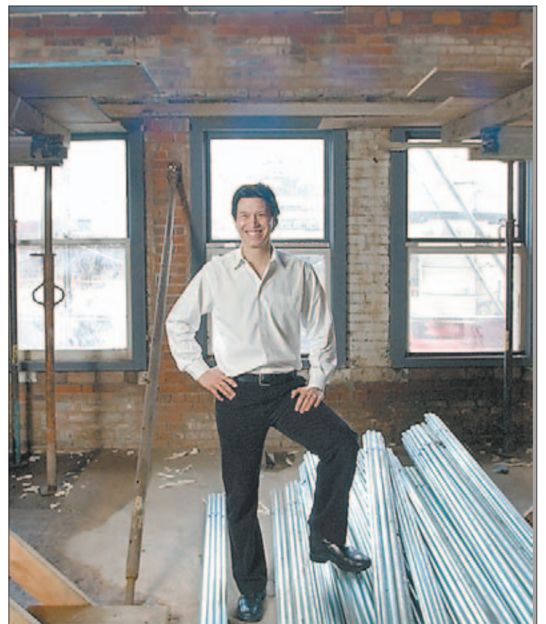
Shown here in one of the lofts he recently introduced into a 100-year-old Beatty Street warehouse, Robert Fung reports that his Salient development group is now preparing to rehabilitate the Flack Block, an 1899 office building at Hastings and Cambie. 'Of special note is that the rehabilitated building will rank environmentally with a LEED 'silver' certification,' he reports. 'This will be achieved through a prudent mechanical and electrical design and the fact that reusing an existing structure inherently reduces the demolition volumes sent to the dump.'
